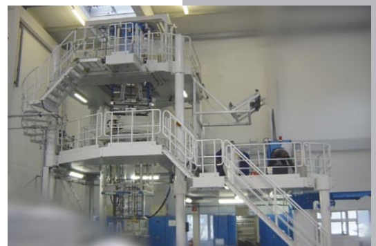
The new extrusion machines of Strubl KG
